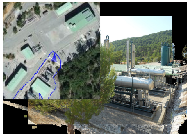
Figure 4: GPS track recorded at Geomethane site The entire the dataset has been georeferenced by comparing the GPS record of the agent who took the pictures with the shot positions estimated by the structure-from-motion pipeline.
